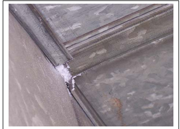
Fig. 1: A look inside sealed ductwork: note buildup of polymer sealant
