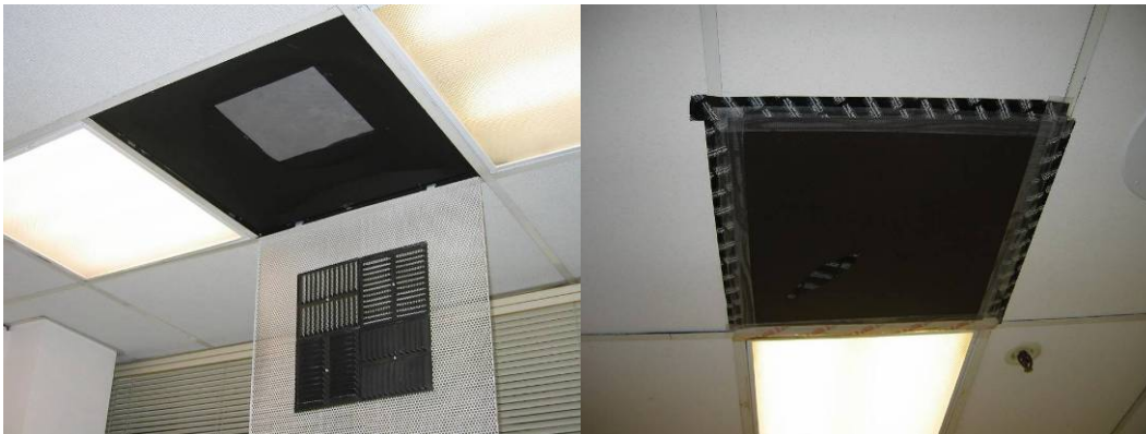
Figure 5: Temporary closure of grilles during aerosol injection. The grille on the left was stuffed with a closed-cell foam plug, whereas the grille on the right was covered with a magnetic sheet and taped at the edges.
