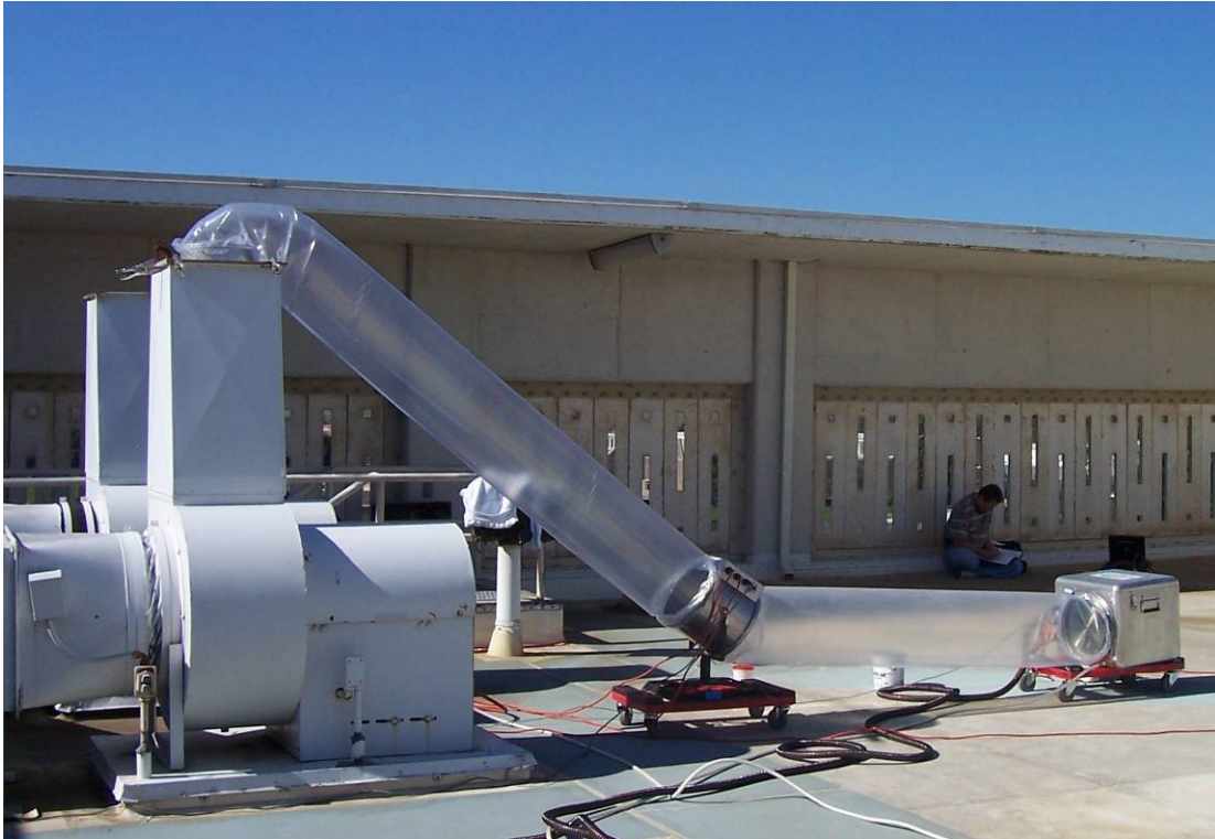
Figure 2: Testing and sealing of exhaust duct leakage at a classroom/laboratory building. Note that the sealant atomizer is installed in the ductwork pointing away from the exhaust fan on the downstream side.
