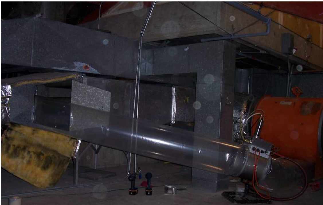
Figure 3: Bachelor's Enlisted Quarters building (i.e. dormitory) being sealed from the penthouse. Note that the sealant atomizer is located outside of the ductwork in the cylinder, and sprays the sealant inside the clear plastic tubing.
