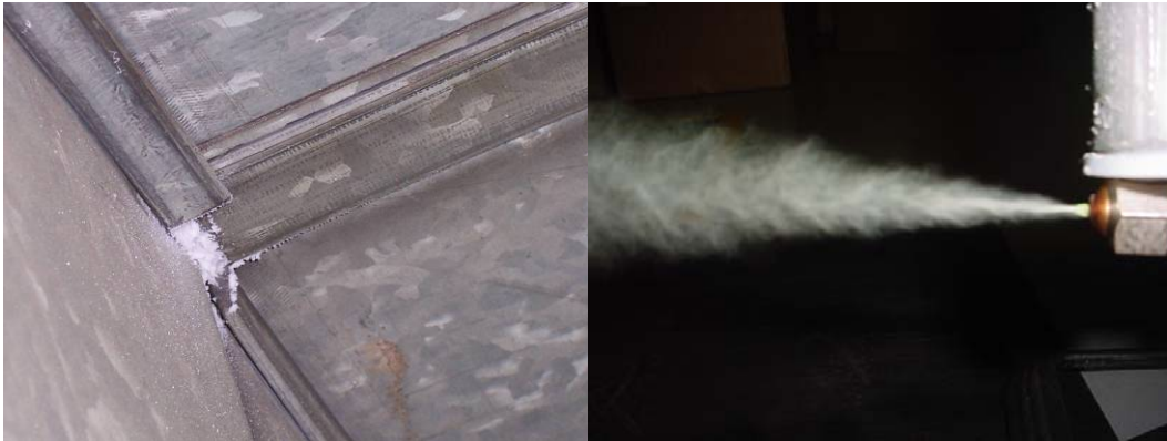
Figure 7: Sealed leak as seen from inside the ductwork, and sealant spray leaving the nozzle. Note that the sealant does not coat the inside of the ductwork, but rather is concentrated at the leaks.
