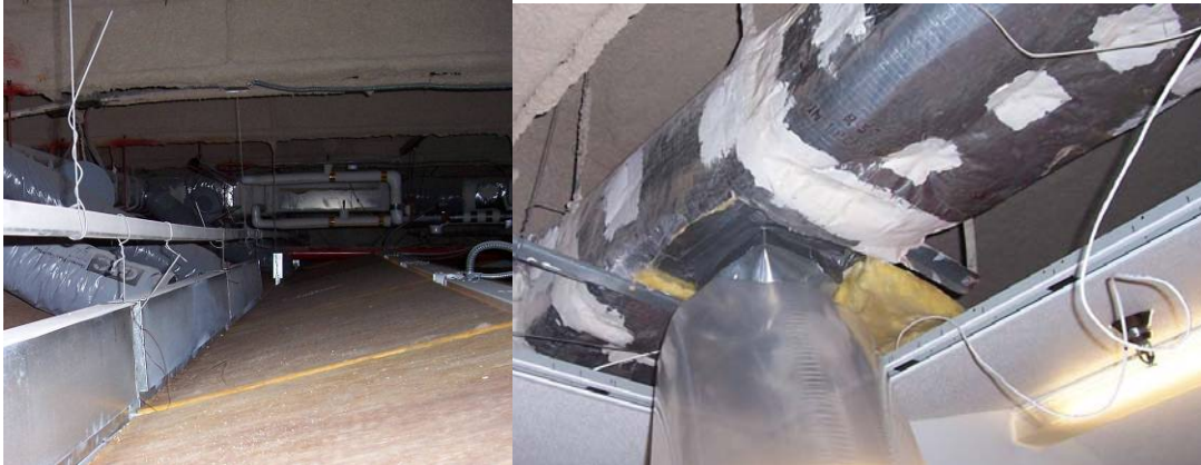
Figure 4: Sealing leaks in an office-building slot diffuser system downstream of VAV boxes. Photo to the right shows one of the injection points used to seal downstream of two VAV boxes simultaneously.
