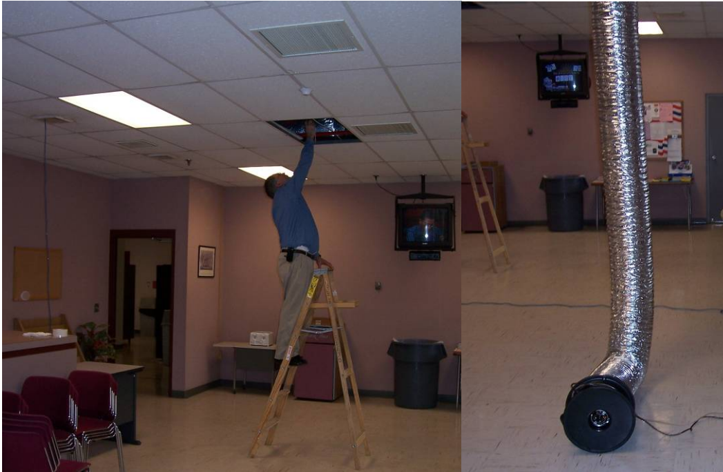
Figure 1: Measurement of leakage downstream of a VAV box in a classroom building. Note duct pressure measurement on left, and calibrated fan on right.
