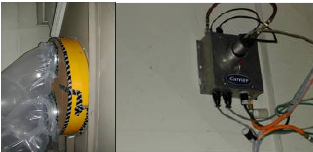
Figure 6: Pressurization through the intake of a 69,000 cfm supply fan for an office building, followed by injection into one of the vertical shafts served by that fan.
