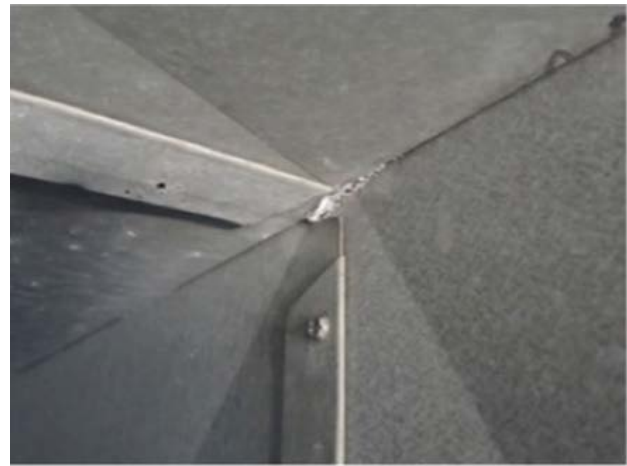
Figure 3: The sealant doesn't coat the duct interior but accumulates only in and around the leaks.
